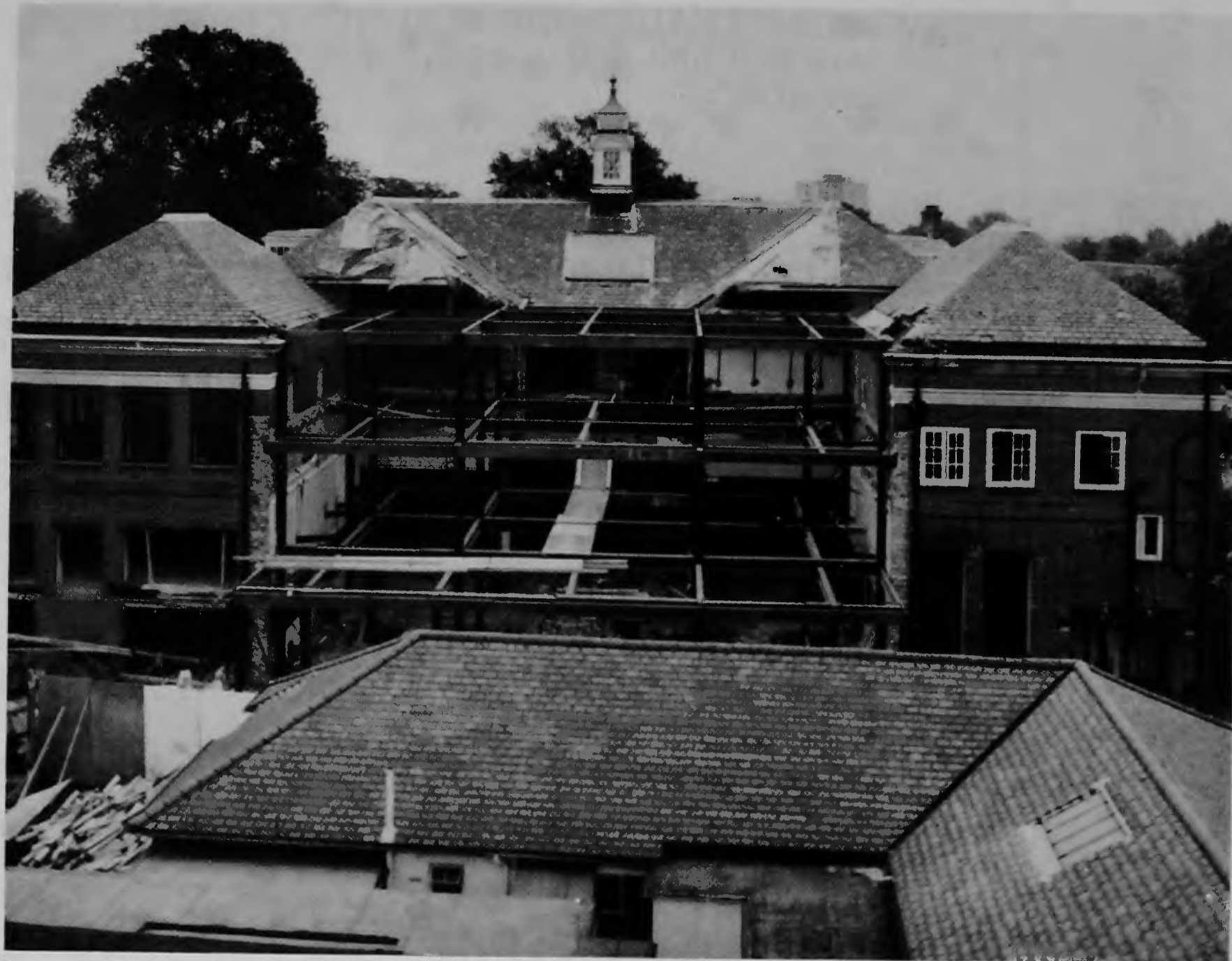
This picture shows the rear of Hendon Library, The Burroughs, where work is progressing well on the major alterations and extensions to the building.
