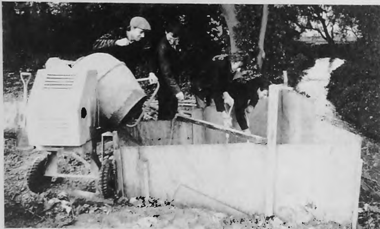
Concreting a bridge abutment to open up a network of paths through Riverside Walk, Whetstone. Left to right, Tim Harwood, John Webb, John Hanratty and Simon Wing.
