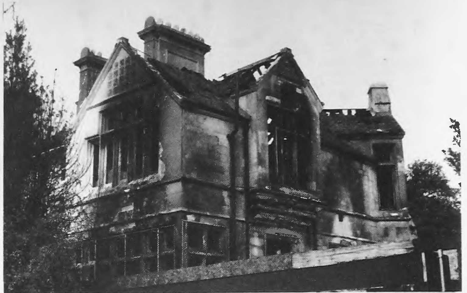
Avenue House after the fire
