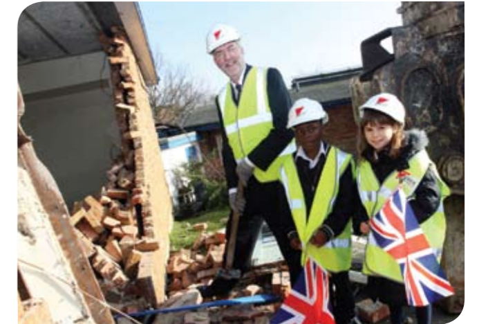
On your marks: Broadfields' pupils Layomi Oladipo and Audrey Linton and teacher Alan King signal the start of the excavation work.
