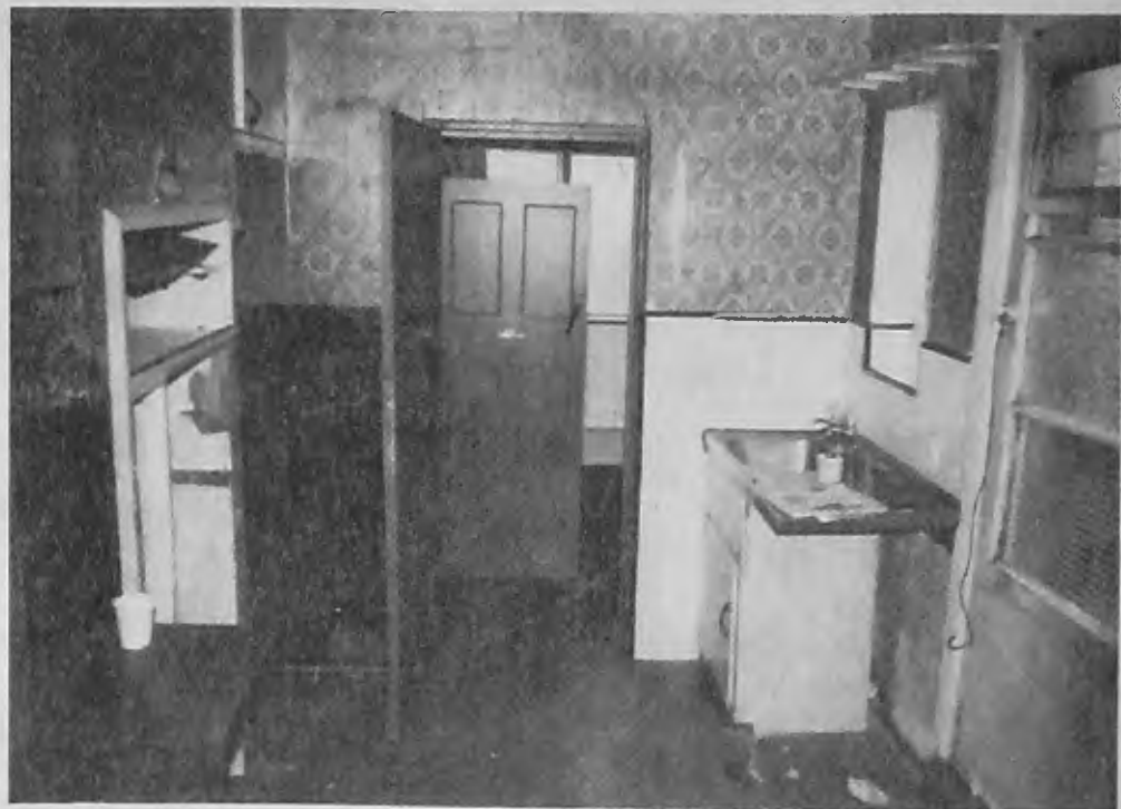
ABOVE: The kitchen at 12 Puller Road as it was before the improvements were carried out.
