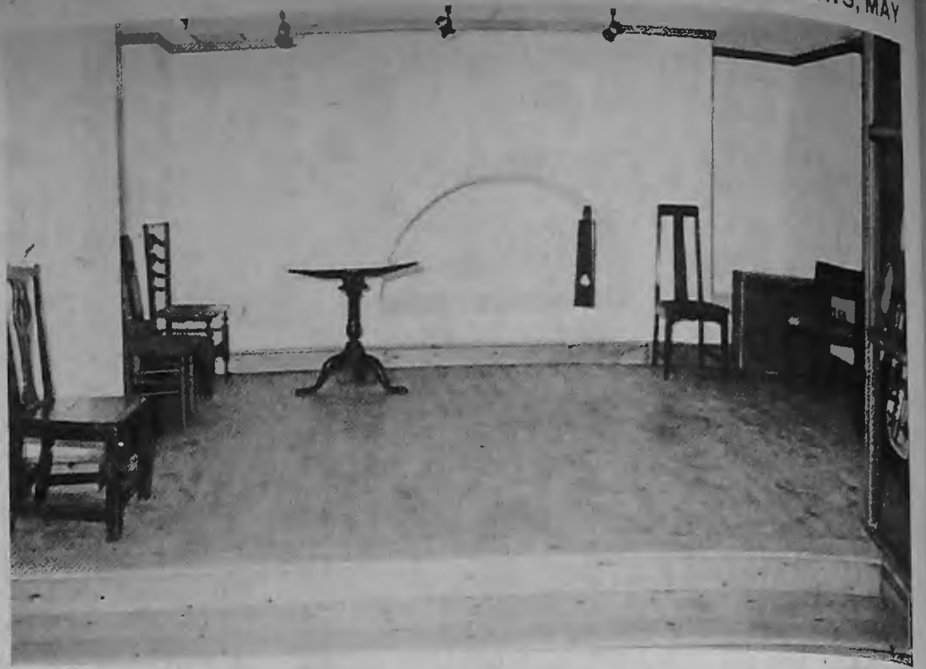
Basement display area with its attractive pine floor and stepped levels which once formed a damp sump.
