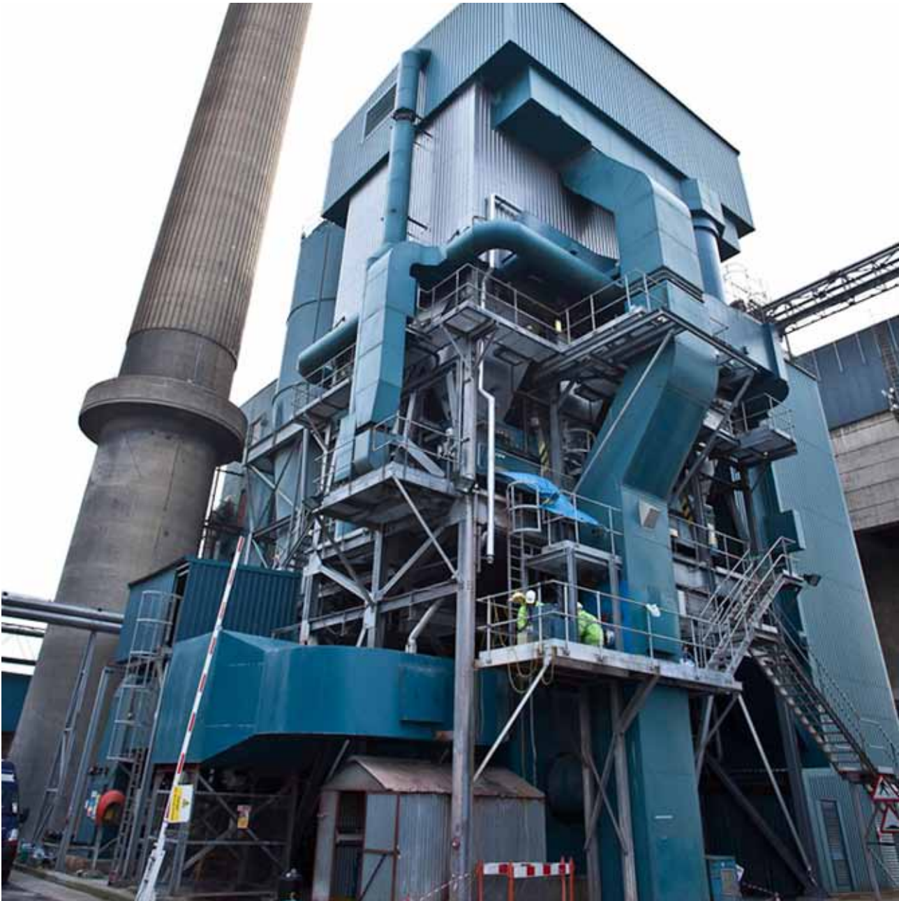
Nottingham Energy from Waste and District Heating Scheme. © CWP Photography
